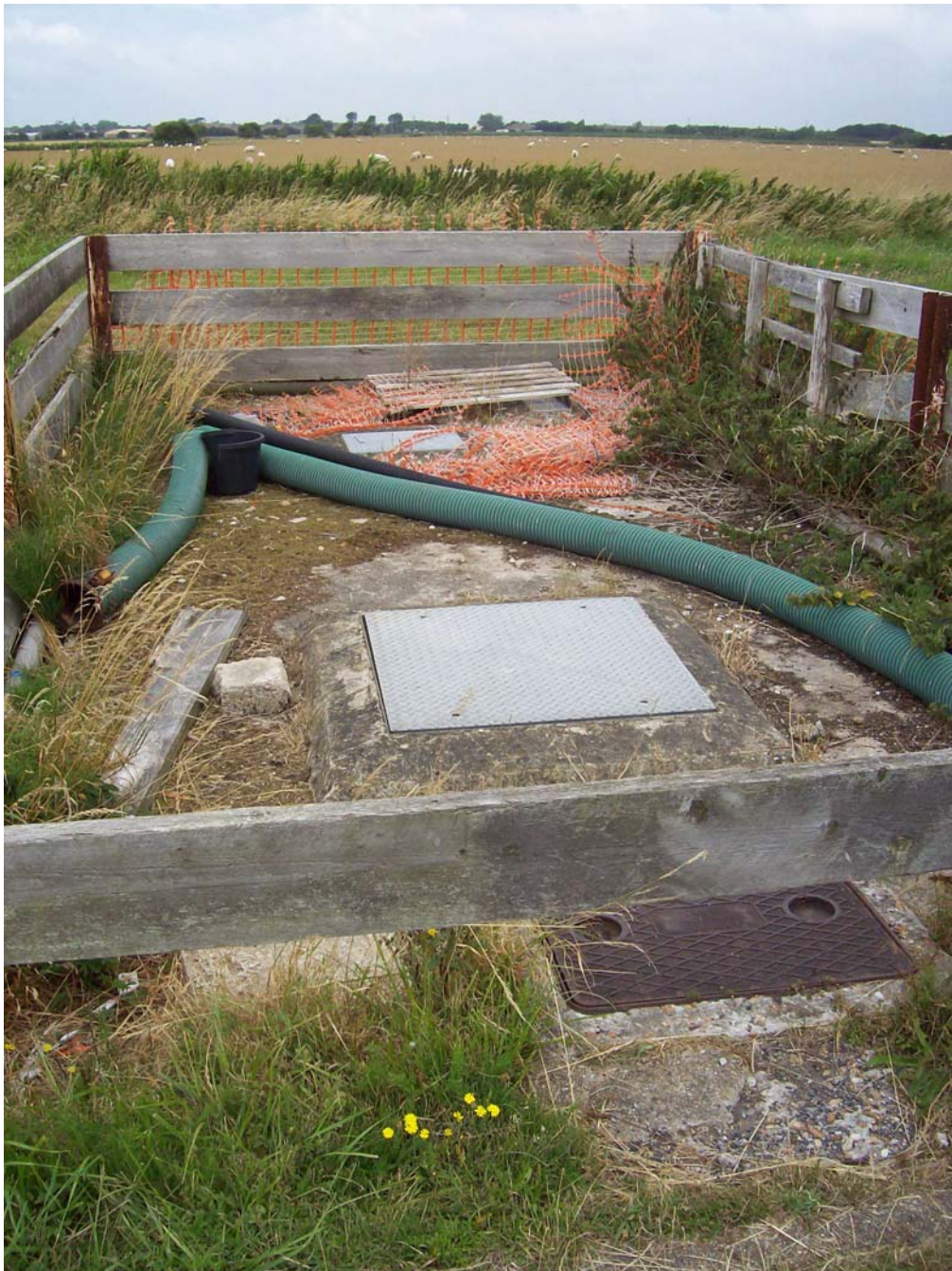
Current septic tank sewage treatment chambers, location adjacent to main car park
